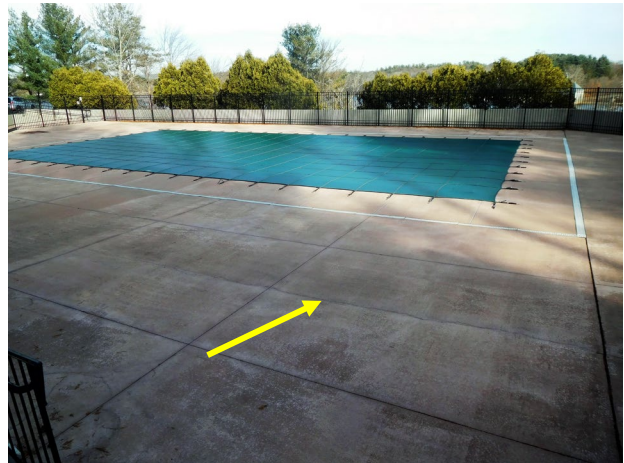
Photograph 3 – View of the pool area with the perimeter metal fence in the background. Note the crack in the concrete pool deck (arrow).
