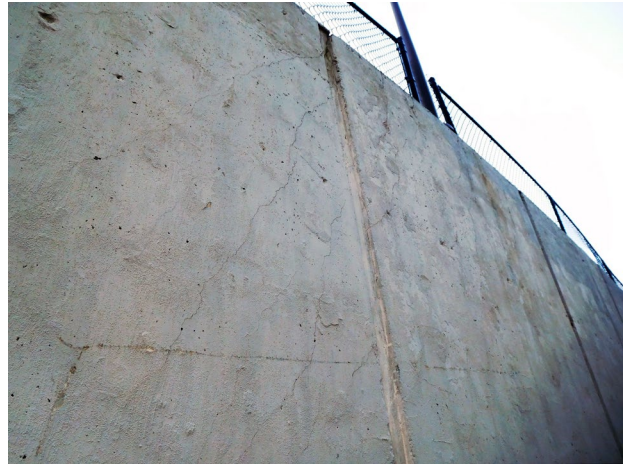
Photograph 7 – Diagonal cracks near the outside corner are indicative of structural deterioration.
