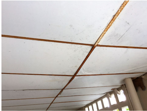
Photograph 12 – Example of a deteriorated garage ceiling area.
